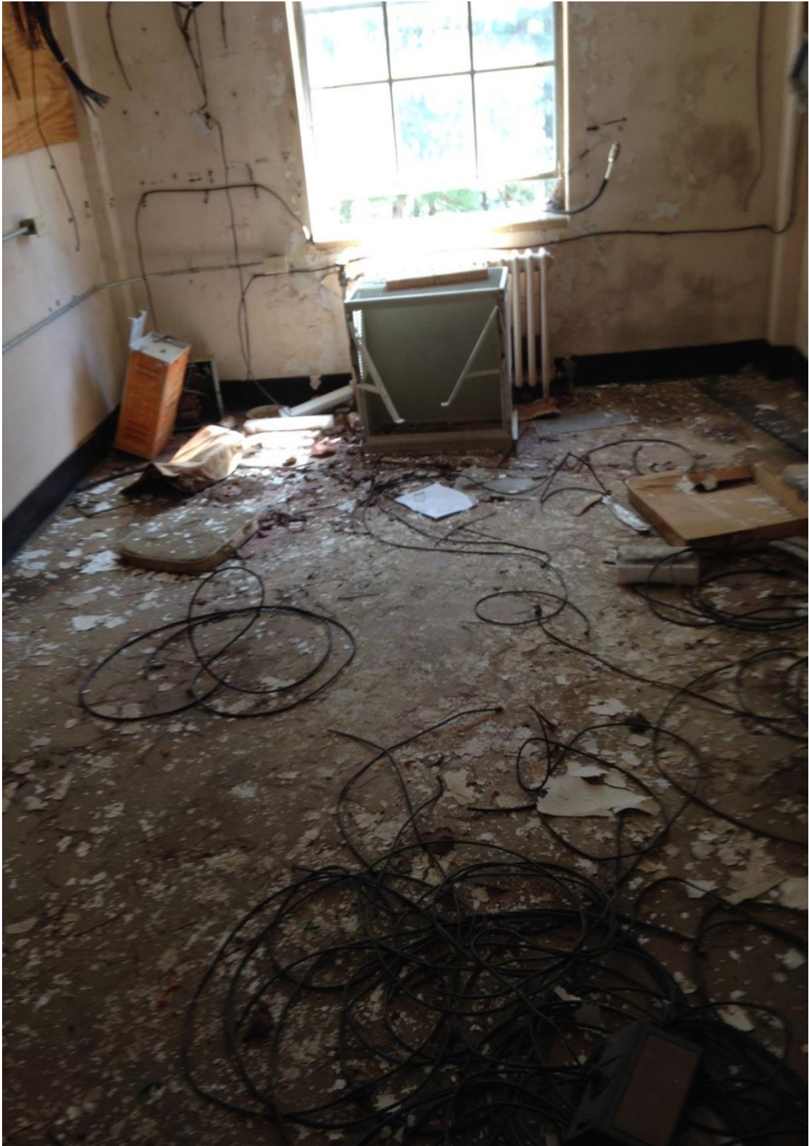
Old Wiring and Debris on the Third Floor of the Hamp Williams Building
