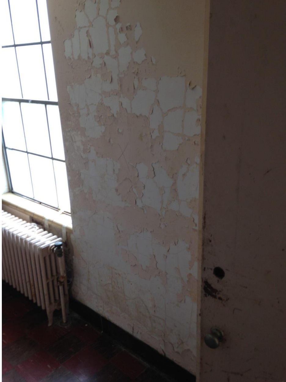
Peeling Paint on the Second Floor of the Hamp Williams Building
