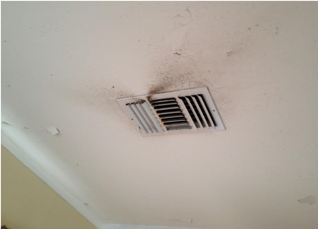
Filth from Cottage Ventilation Duct
