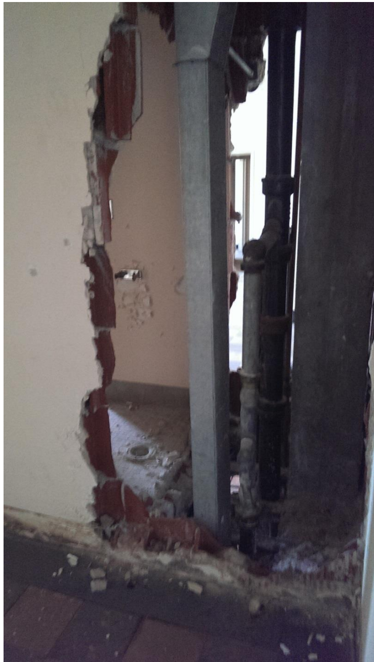
Damaged Walls and Debris on the Third Floor of the Hamp Williams Building
