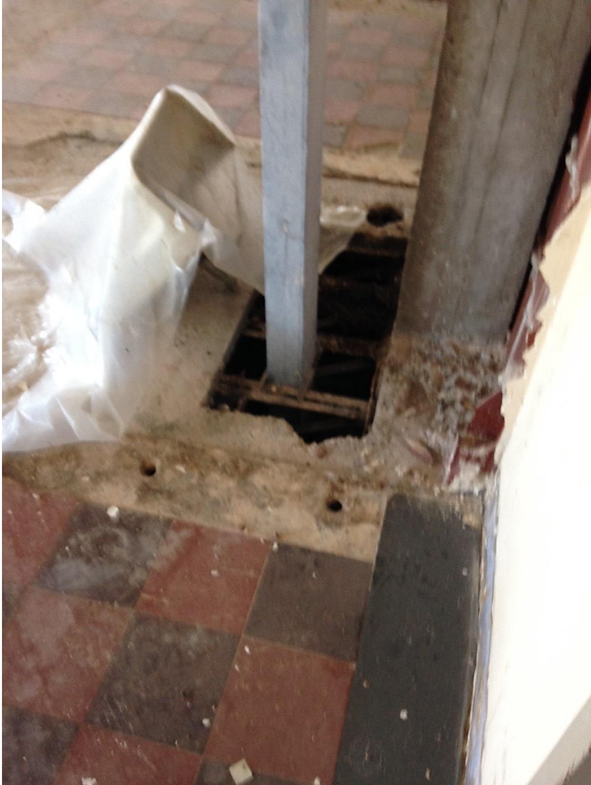
Holes in the Floor on the Third Floor of the Hamp Williams Building
