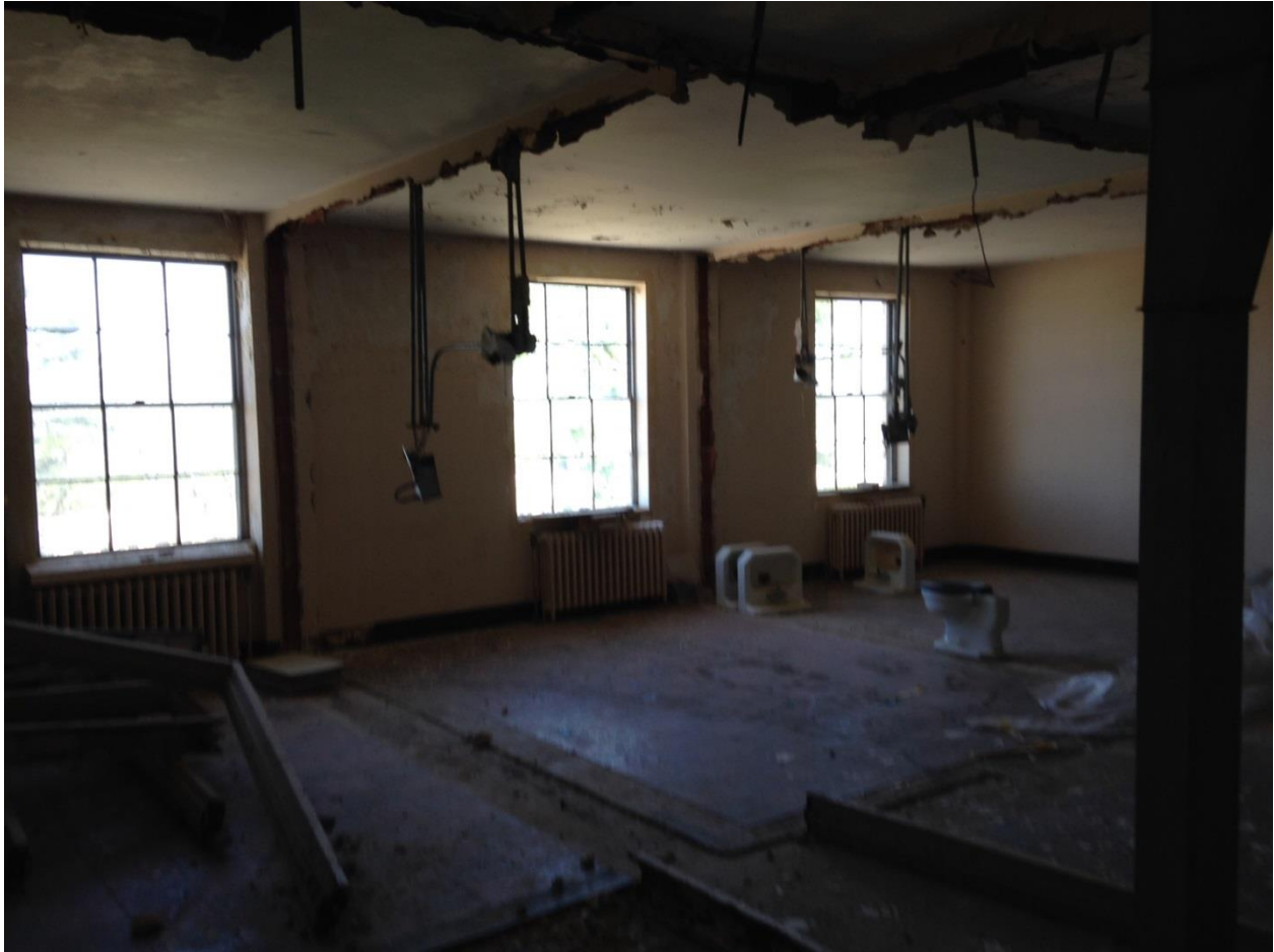
Missing Walls and More Debris on the Third Floor of the Hamp Williams Building
