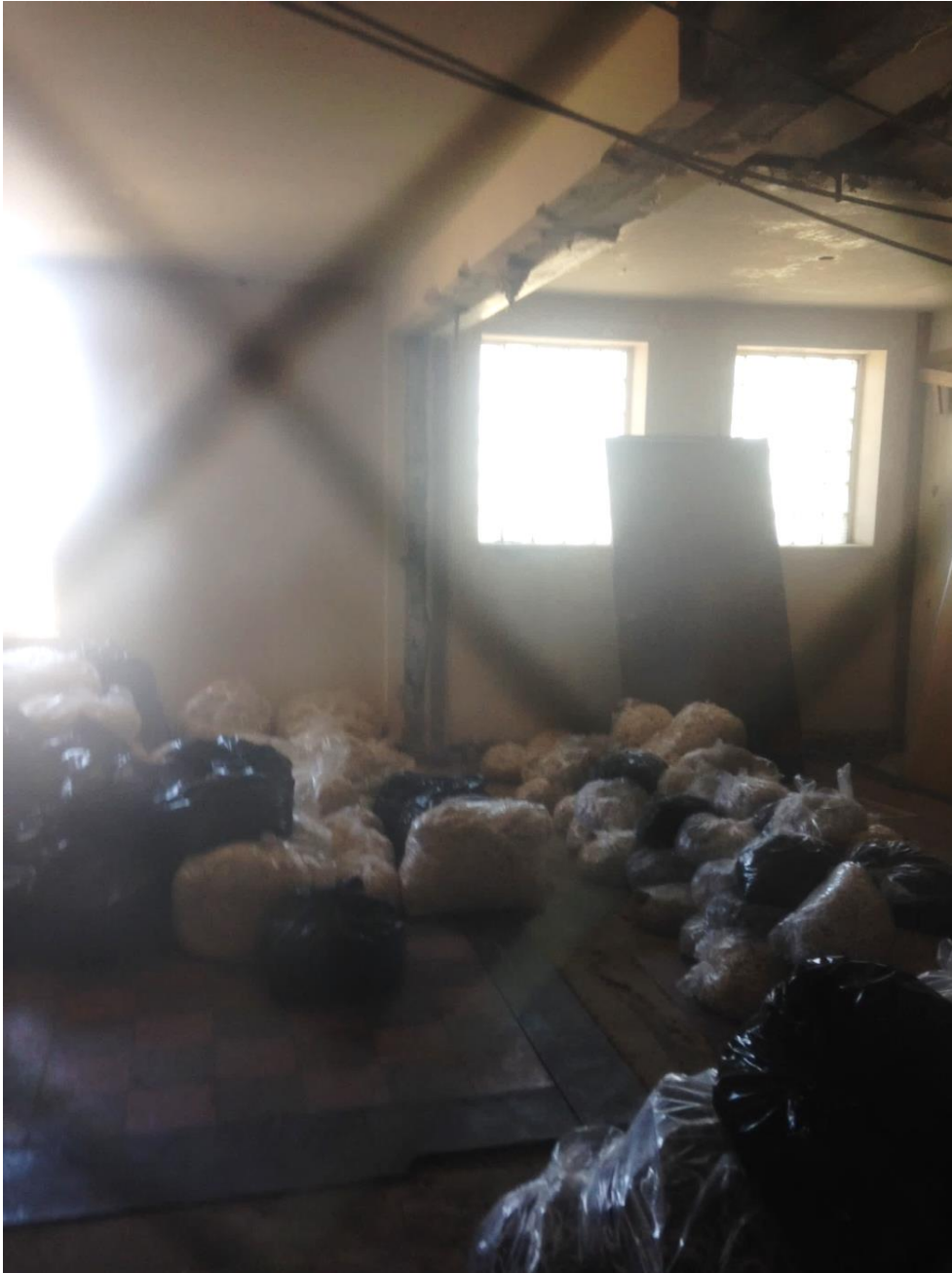
Trash and Debris on the Second Floor of the Hamp Williams Building
