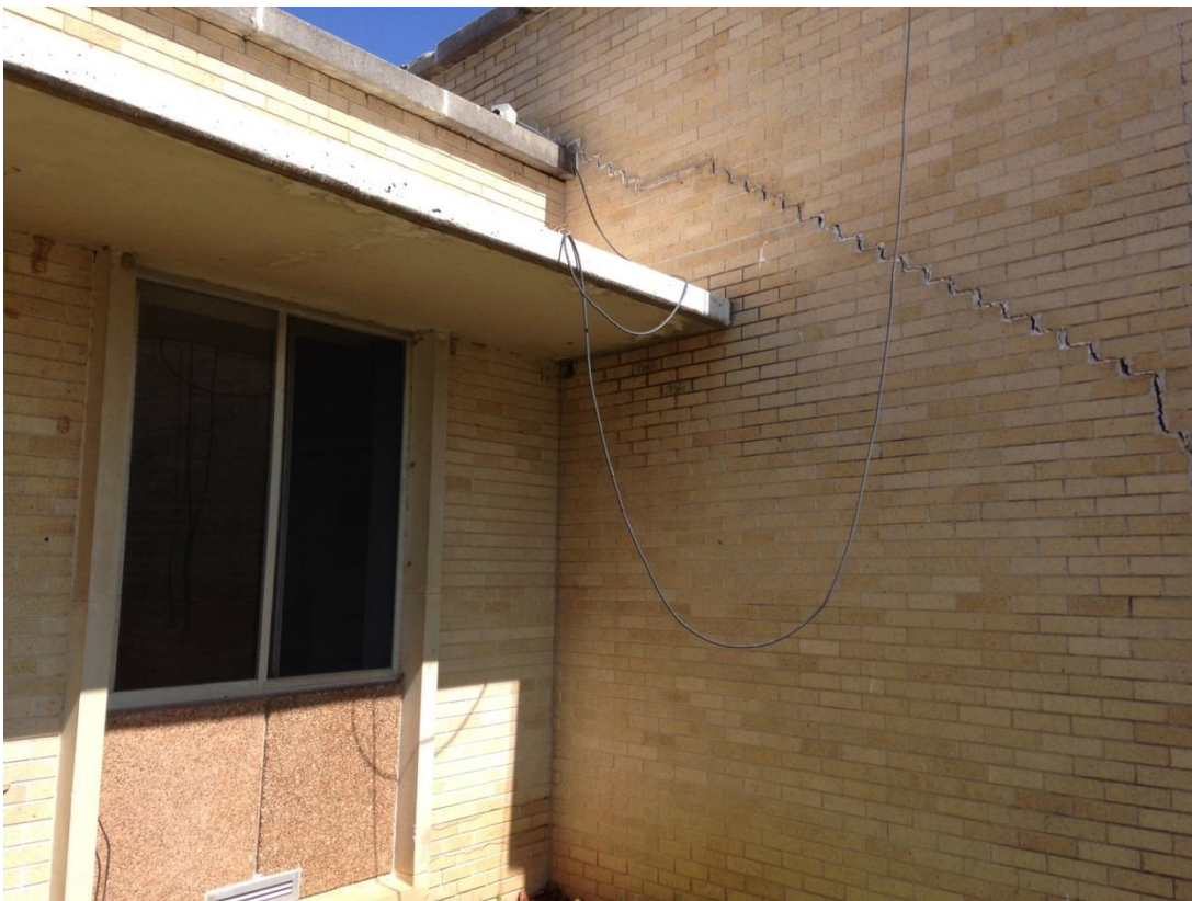
Exterior of the Judge Hill Building Showing Need for Repairs
